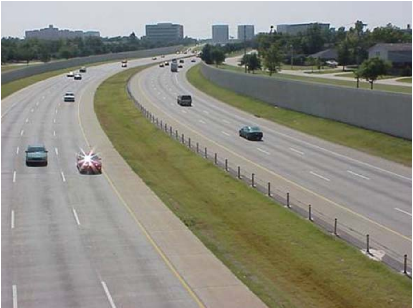
Photograph of cable barrier in the median of a roadway
